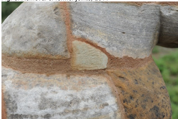
Fig. 5: Pointed joints while wet, 2011
