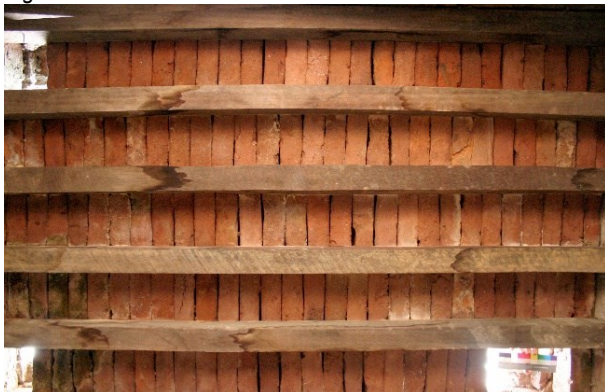
Fig. 10: Former seating, loose bricks / wooden beams
