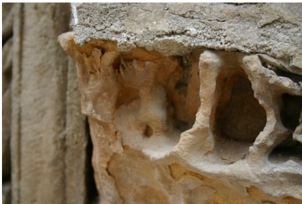
Fig. 12: Detail of extremely weathered carved stone and cement joint (upper part)
