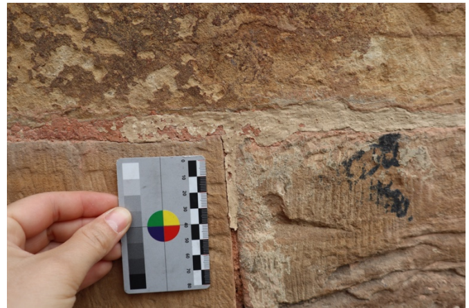
Fig. 9: Powdering of joint retouching revealing pinkish joint mortar.
