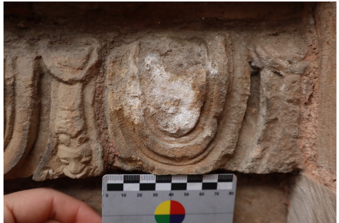
Fig. 7: Salt efflorescence causing material loss.
