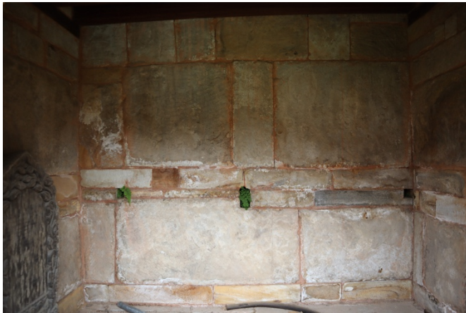
Fig. 6: Salt efflorescence on the inside of the pavilion base.
