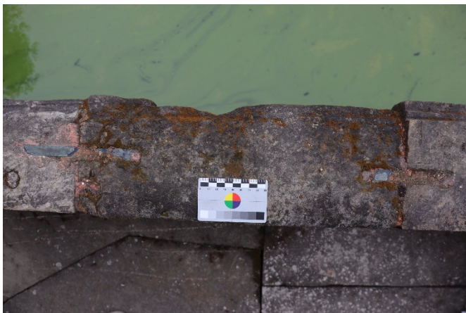
Fig. 10: Inox pins at the balustrade with chipped off mortar.
