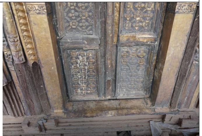
Fig. 10: Door covered in dust from construction work, May 2024
