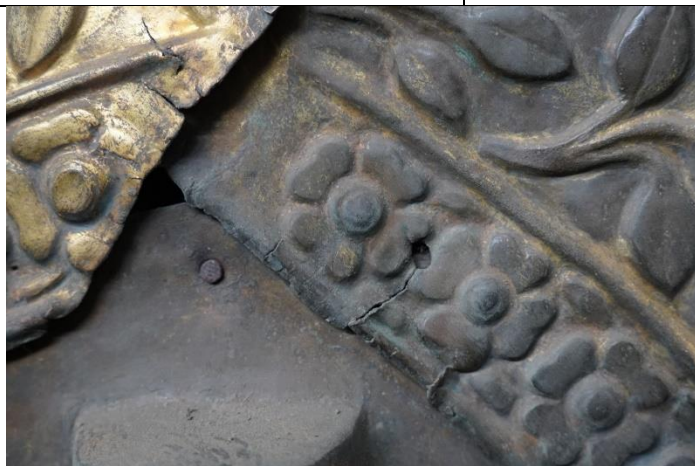
Fig. 16: Cracks in the Torana's copper sheet repousse, May 2024
