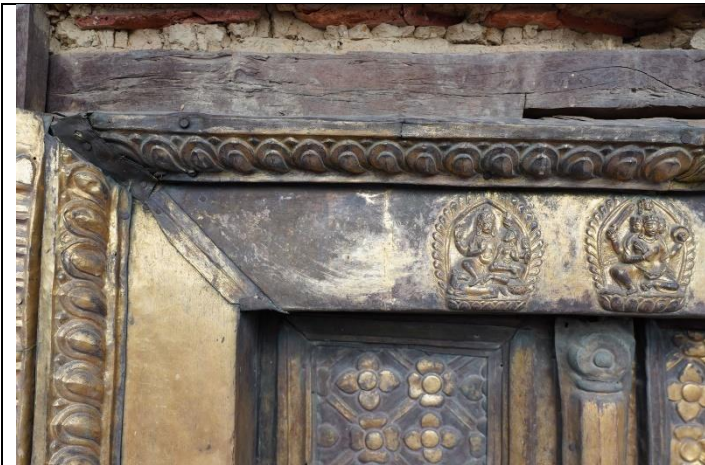
Fig. 7: Abraded areas / worn out gilding on the upper frame of the door, May 2024
