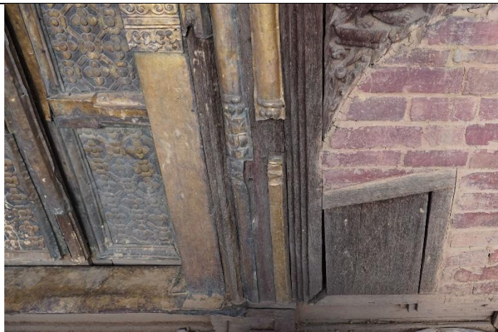
Fig. 3: Missing elements in the lower area of the door, May 2024
