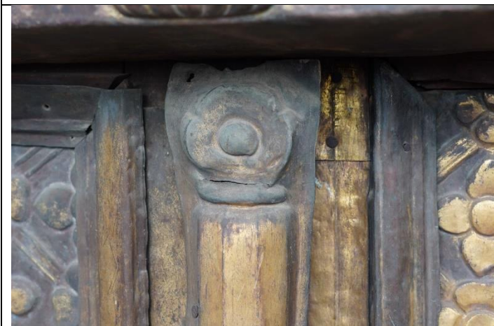
Fig. 9: Partial green corrosion on some door elements, May 2024
