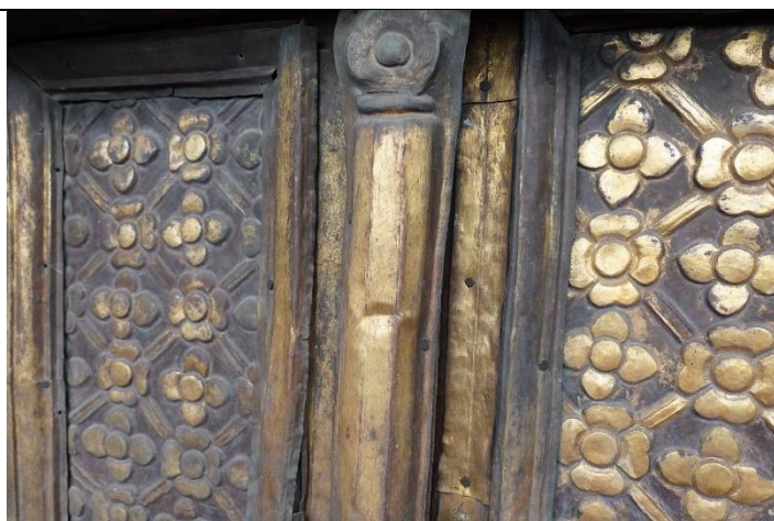
Fig. 5: Deformation on the baffle plate in the centre of the door, May 2024
