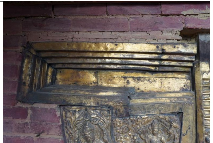
Fig. 8: Abraded areas / worn out gilding on the copper sheet repousse on the sides of the door, May 2024
