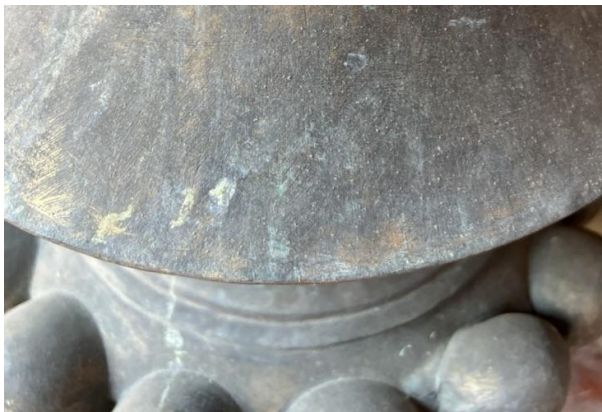
Fig. 7: Soiled and corroded surfaces
