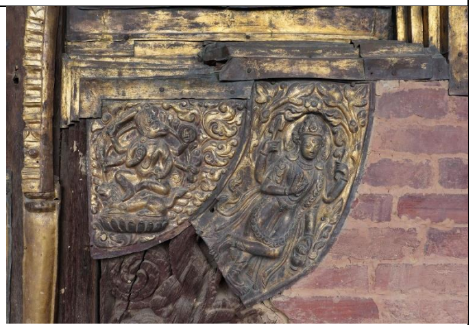
Fig. 6: Abraded areas / worn out gilding on the copper sheet repousse on the sides of the door, May 2024
