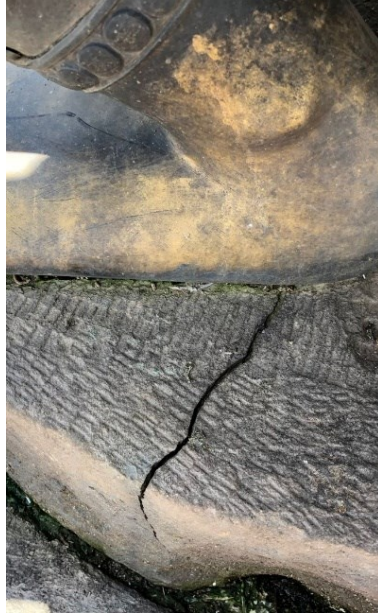
Fig. 11: Crack at the plinth
