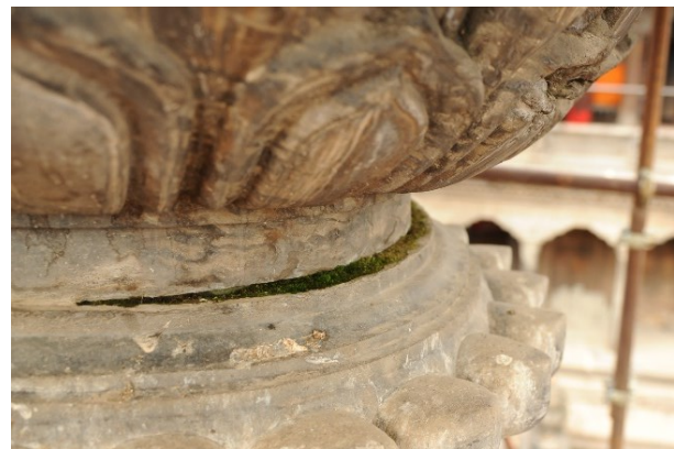
Fig. 9: Moss growth within joint
