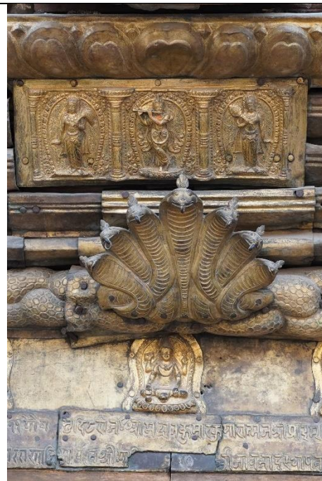
Fig. 15: Missing decoration-elements ( naga mouths)
