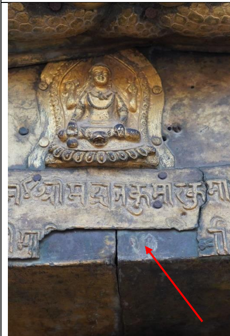
Fig. 14: Missing inscription (red arrow) and nails as well as cracks on the upper door wing
