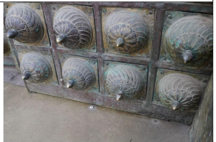
Fig. 29: Green corrosion on lower area of the right doorwing
