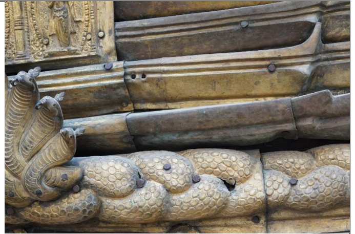
Fig. 31: Corroding iron nails on snake ornament and kulām
