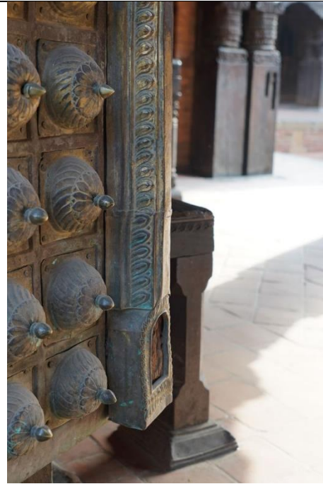
Fig. 38: Green corrosion on the lower area of the baffle plate
