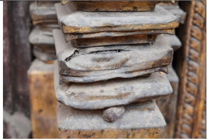
Fig. 29: Deformations and dust accumulations on the left pillar
