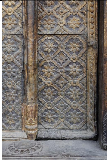
Fig. 15: Cracks and deformations on the right lower door wing and baffle plate
