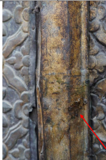
Fig. 31: Soiling on the baffle plate
