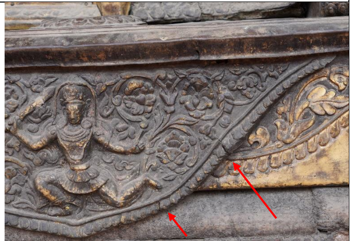
Fig. 14: Cracks close to the Durga figure
