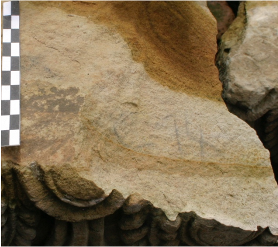
Fig. 1: Visual inspection of the sandstone from Bhandarkhal Tank Pavilion Base, © IoC 2010.
