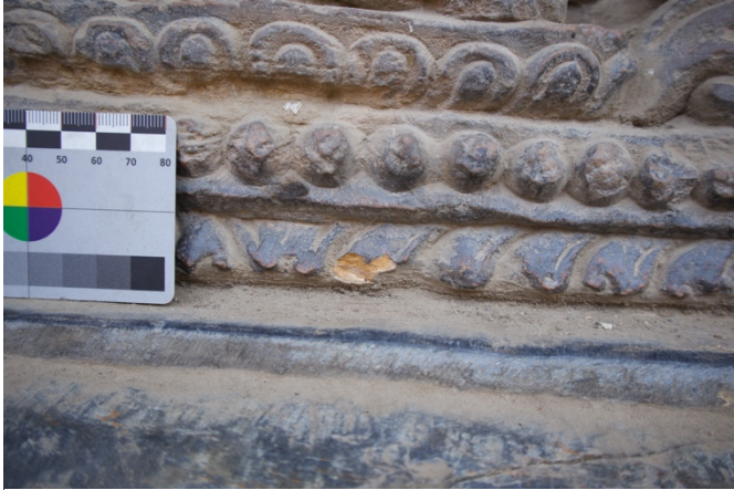
Fig. 2: Material loss due to salt efflorescence.
