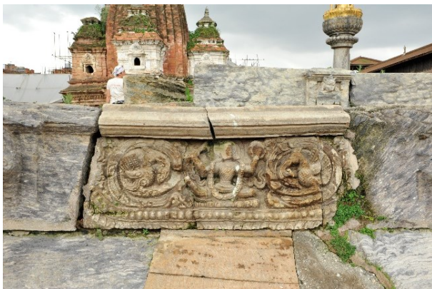
Fig. 14: Totally cracked figurative block, 2017
