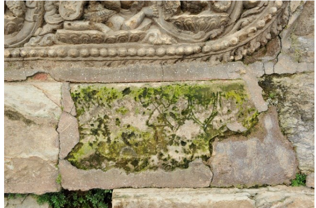
Fig. 19: Insufficient cement joints incl. algae, 2017
