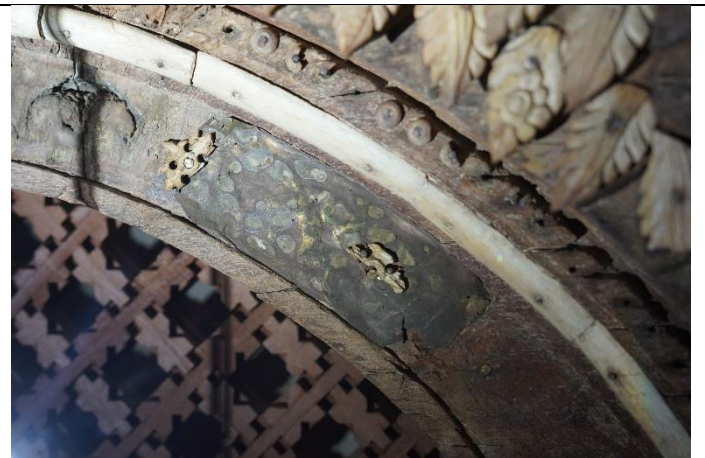
Fig. 10: Green corrosion on the copper sheets with almost all the gilding worn out, May 2024
