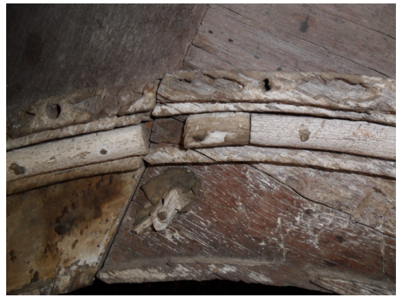
Fig. 12: Loose and missing parts, visible fixing
