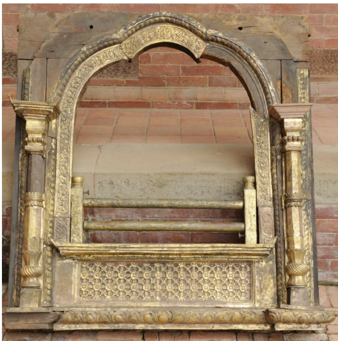
Fig. 32: Overview of the preserved metal window without reconstructed parts before integrating in the ensemble, 2013
