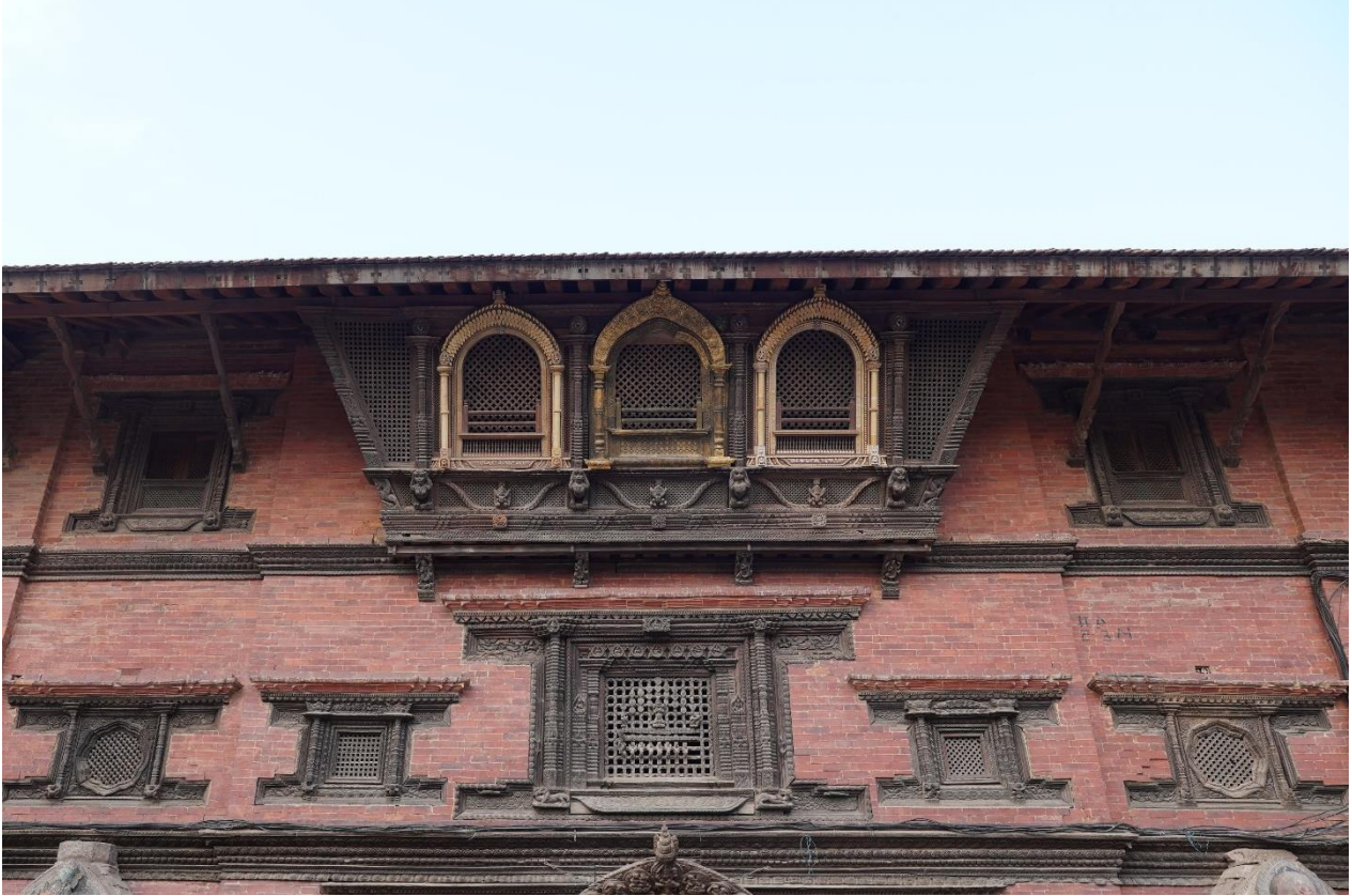
Fig. 1: Golden window and reconstructed ivory windows on the facade of Sundari Chowk, May 2024
