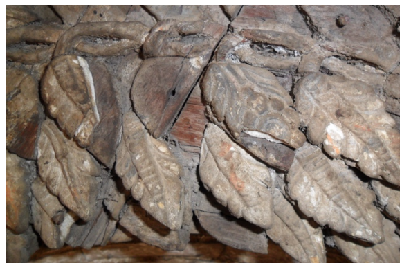
Fig. 14: Wooden Support after dry cleaning, 2013
