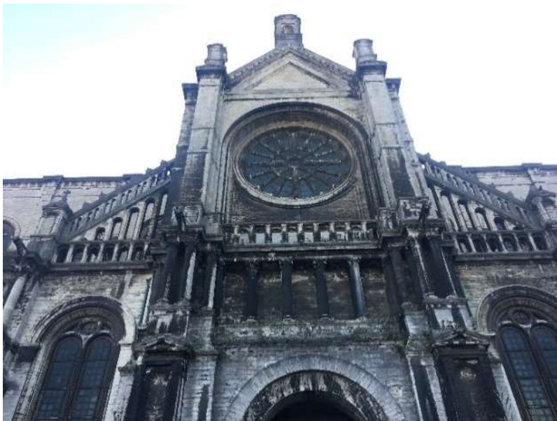
Fig. 21-23: St. Katherina church in Brussels: sulphation crusts (left up and down) and the half-cleaned façade (right)
